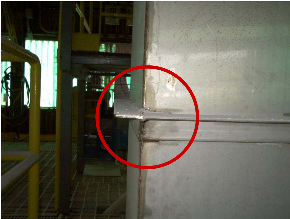
Figure 3-2. A flat surface that can collect product (This should be eliminated or sloped).
